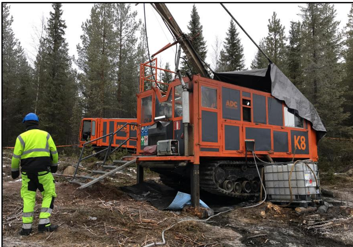
Figure 12.1 – Photograph of drill rig visited by the author during the site visit
